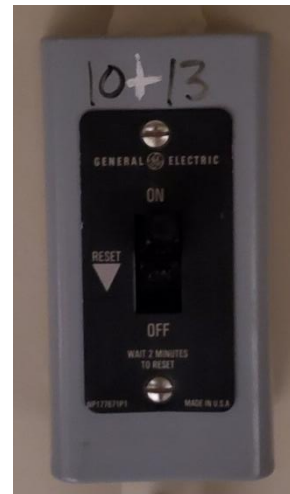
Figure 1.8 Extractor fan switch
